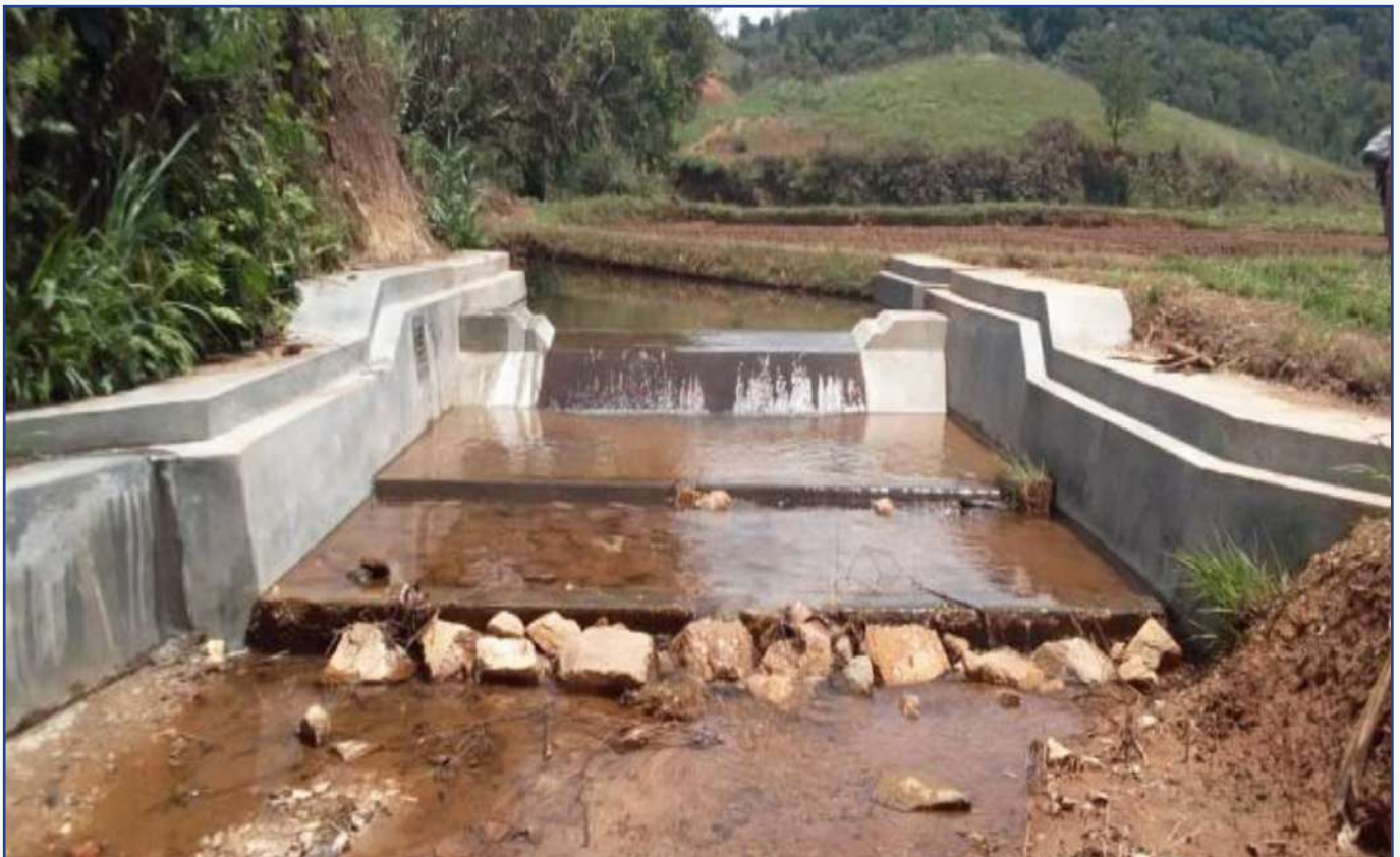
CC Head Water Dam under Them Lawbyrtun Cluster-I RIDF-XXIV, Wahskei, West Khasi Hills
