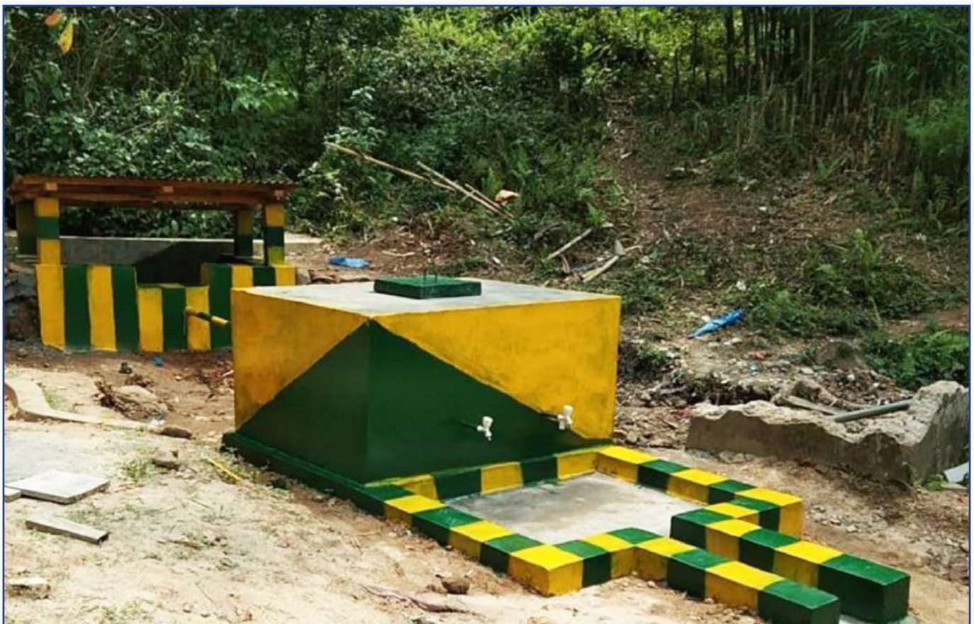
Spring-Chamber with Storage Tank
